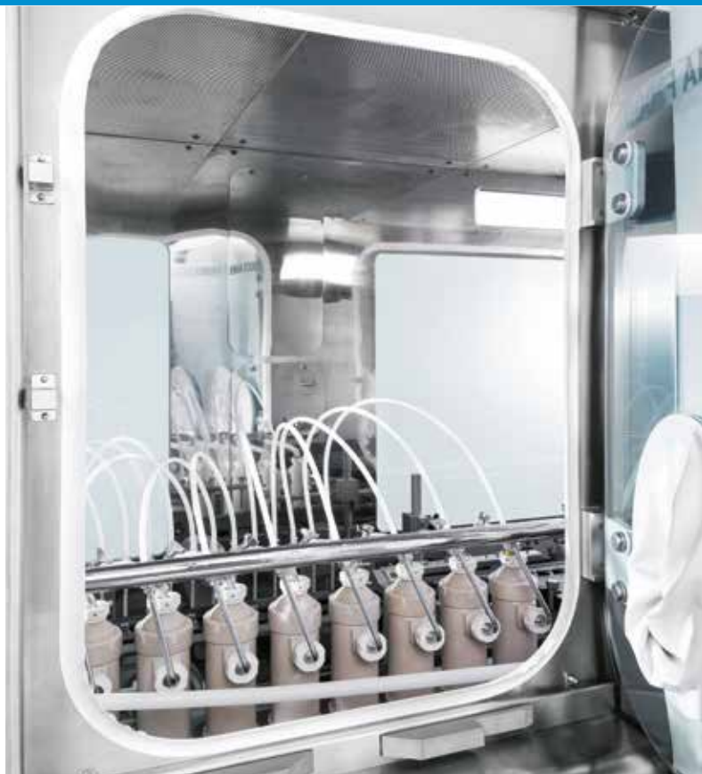
Gaskets and details of filling area
